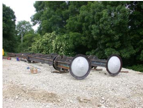
Installation of O-cells and pressure cell on the bottom of the carrying frame
