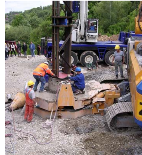
Installation of the O-cells on the steel carrying frame into the pile bore
