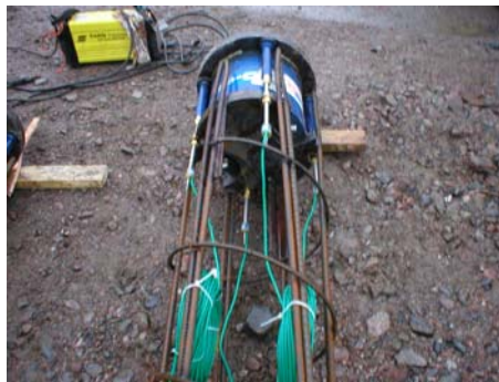
O-cell® test assembly welded to steel hanging cage prior to installation into the driven steel tube.
